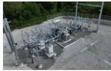
Substation at the Jeannette plant
